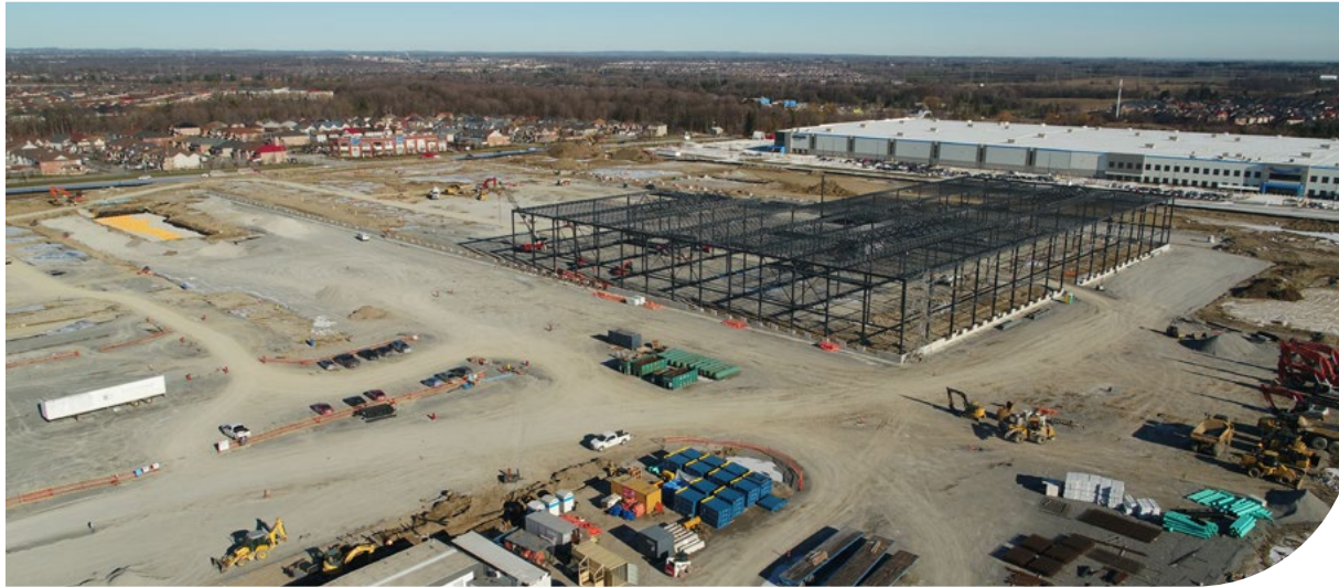
January 2021 photograph shows our new leading-edge Ontario East Processing Centre under construction in northeastern Toronto. A storm water management storage chamber is at the top left.
